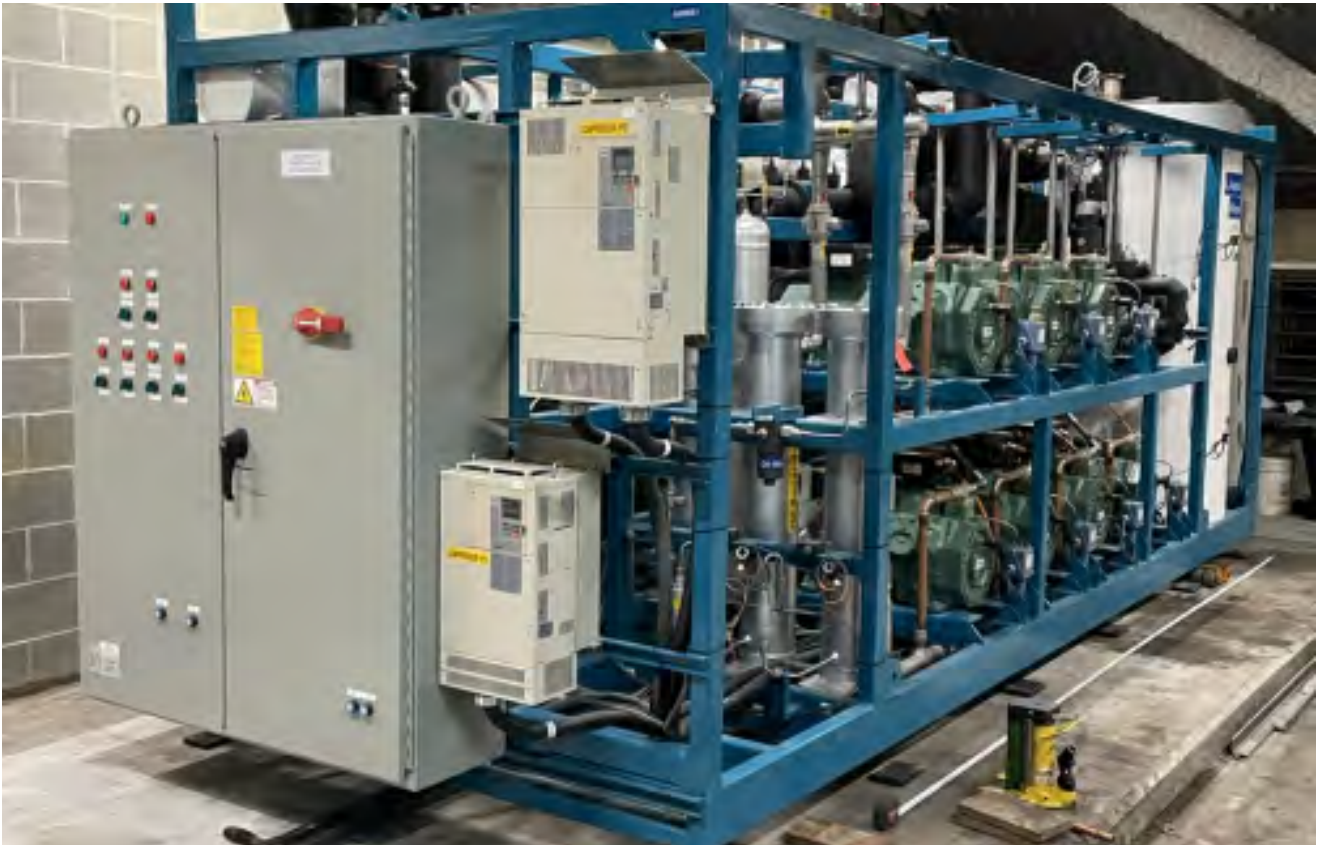
CO 2 package at Santander Arena; Nationwide Arena will install two similar packages in 2023.
