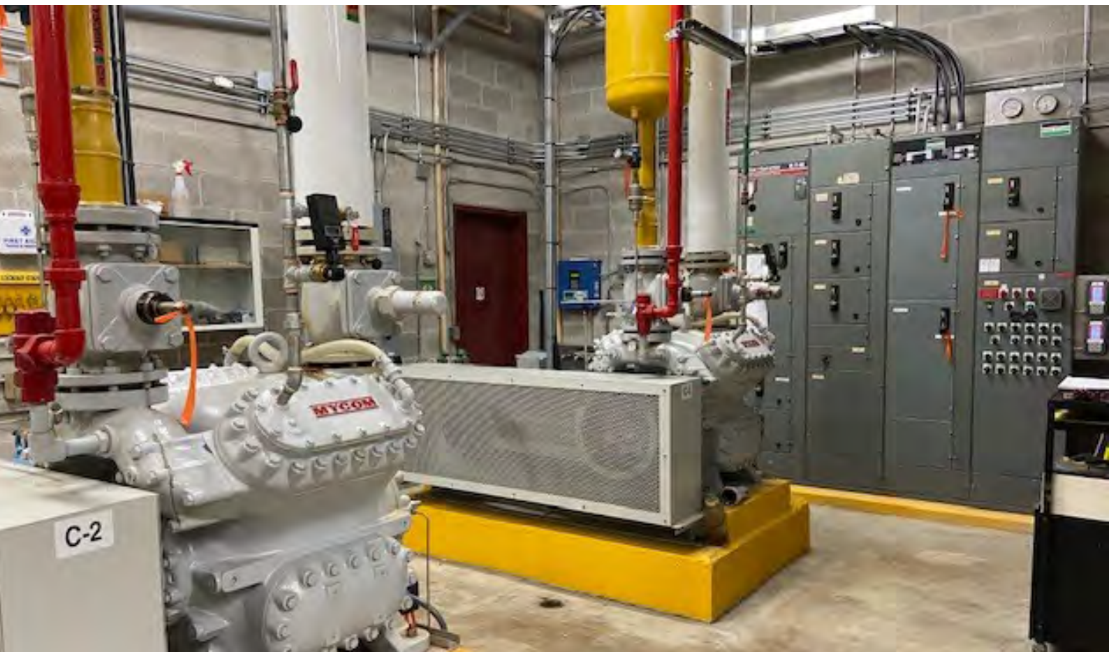
Compressor room, Pickering Ice Arena
