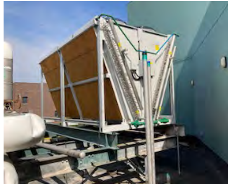
CO 2 gas cooler at Santander Arena; Nationwide Arena will install the same model in 2023.
