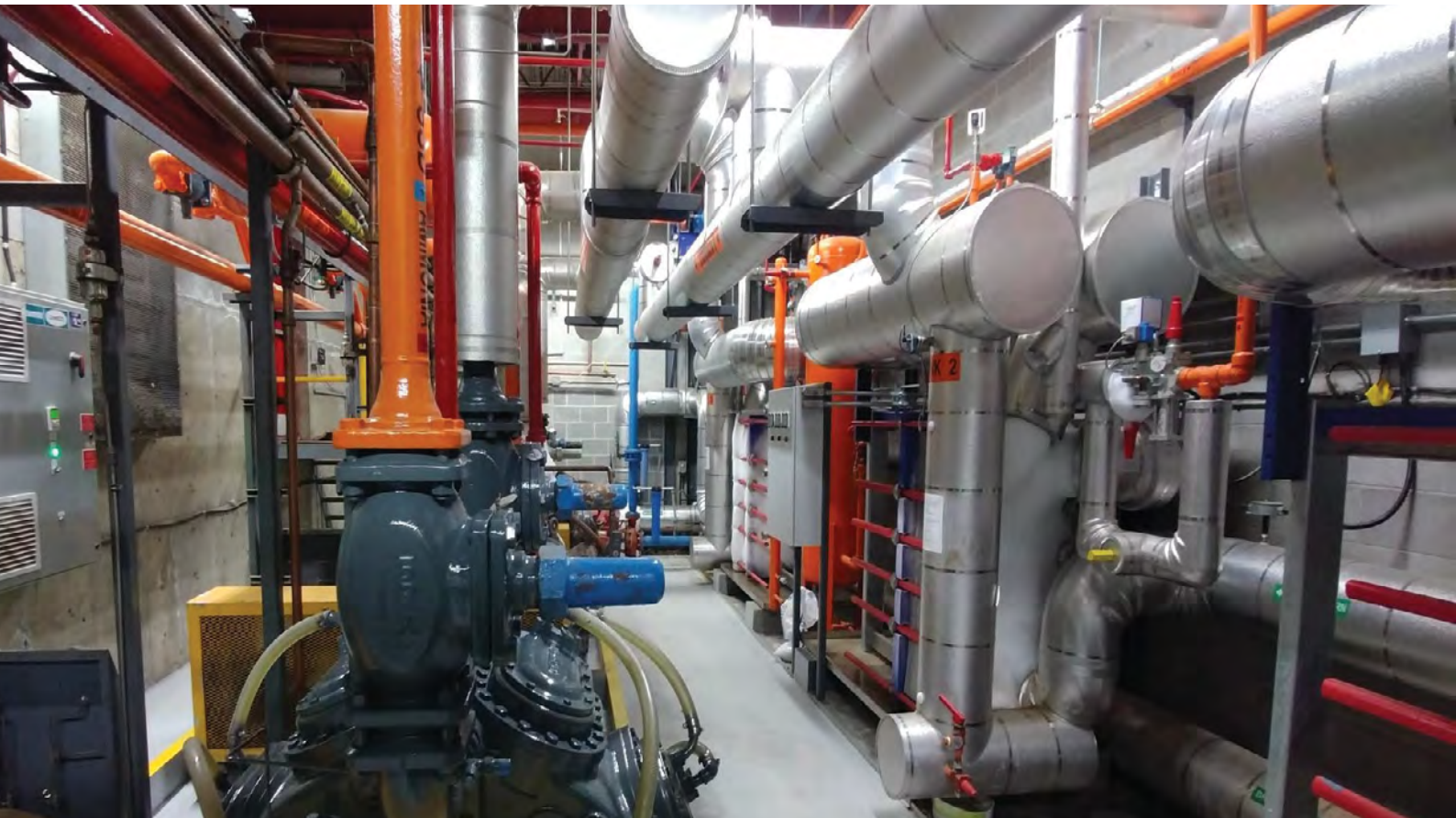
U-Turn installation in Canlan Sports arena Burnaby EightRinks
