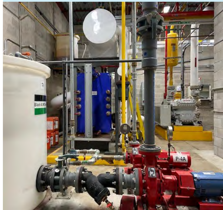
At left: white evaporative condenser water tank; at middle, rear: blue plate-and-frame heat exchanger, Pickering ice arena.
