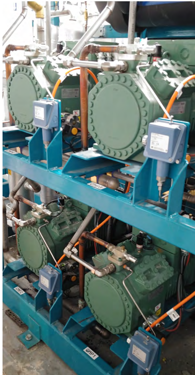
CO 2 rack at Centre Sportif Sainte-Anne-Des Plaines
